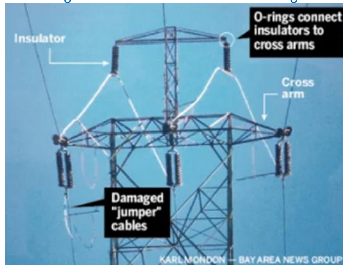
Figure 1: Powerline Transmission Latticing
